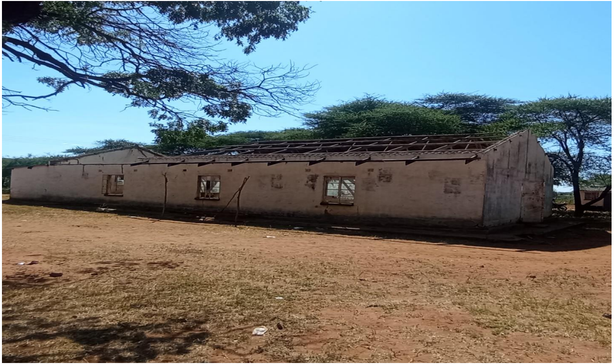
Figure 52: Dilapidated Manoti Community Hall
